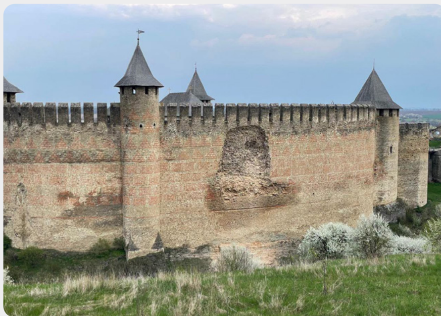
Collapse of part of the wall of Khotyn Fortress Source: BukInfo .
